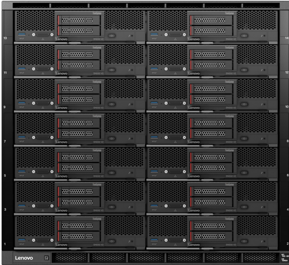
Figure 6. ThinkSystem SN550 V2 servers installed in the Flex System Enterprise Chassis The SN550 V2 server is supported in the Flex System chassis as listed in the following table.
